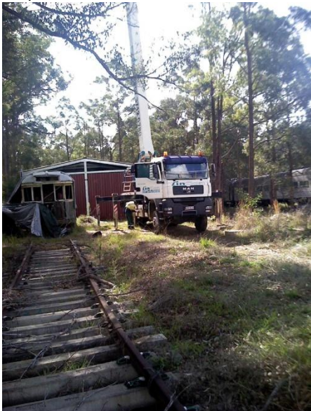
Photo: Optus with a 40m cherry picker looking at new site behind shed.
